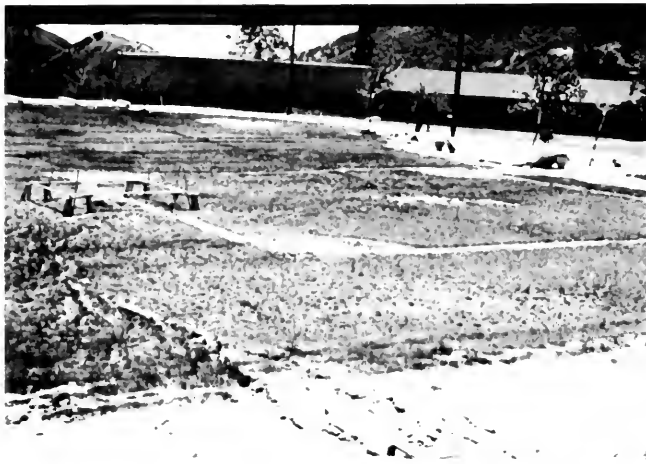
Photo 19. Ground cracks associated with failure of materials (alluvium) under fill materials.
